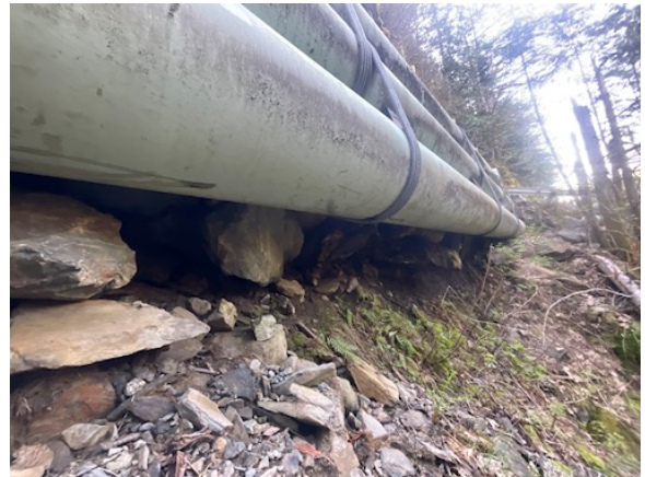
Foundation being undermined with coarse road fill visible.
