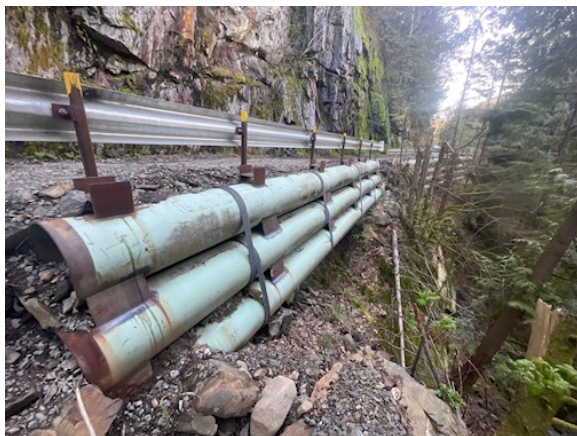
Wall facing (pipe and cable leash) with steel guard rails
